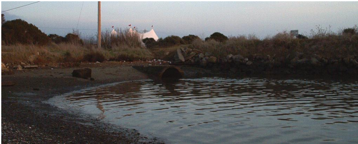
The Virginia Street storm drain system outlet channels Schoolhouse Creek waters into the Bay.
